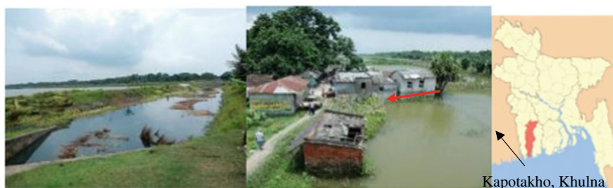
Fig. 14.6 Poor polder drainage (left) and sedimentation resulted in inundations marked by levels of discoloration in buildings (middle) (Kapotakho in Khulna District, 2014)
