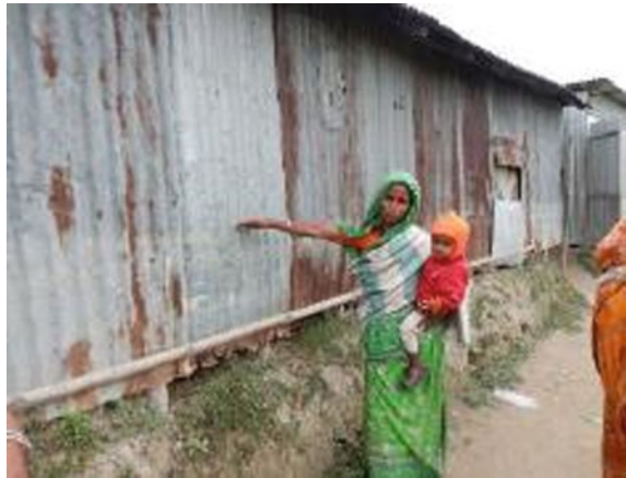
Fig. 14.11 Houses on plinth. A woman shows the height of the recent flood (Sundarganj District, Gaibandha Division, 2014)
