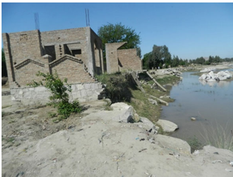
Fig. 18.3 Riverside community in Bihsud District in Nangahar Province. Recurrent floods affect the community and erosion of river bank poses a significant threat (photo provided by CWS Japan)
