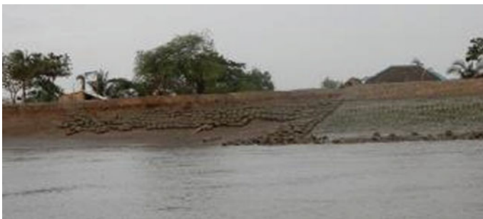
Fig. 14.12 Sand bags and concrete blocks are placed on the embankment to prevent erosion (Fulchhari District, Gaibandha Division, 2014)
