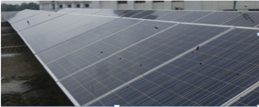
Fig. 23.1 String of 50 KW system situated at university roof
