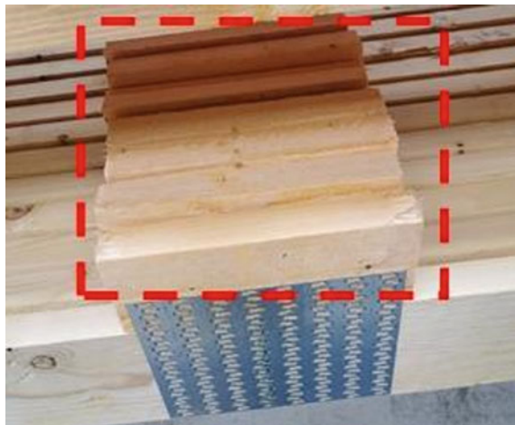
Fig. 14 Highlighted dashed box illustrates the timber packers to compensate for the plate which is too large for fixing timber elements together on the roof truss (author image 2019)
