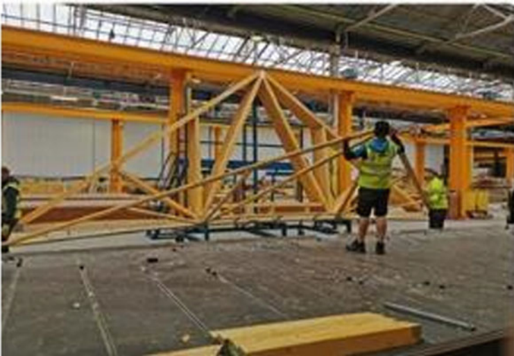
Fig. 5 (Right)—Completed truss being lifted off the press bed and onto the rack
