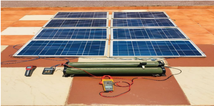
Fig. 8 Field setup for proposed solar PV network at the rooftop
