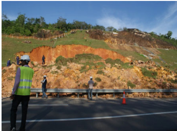
Fig. 15.25 Failed slope at southern expressway
