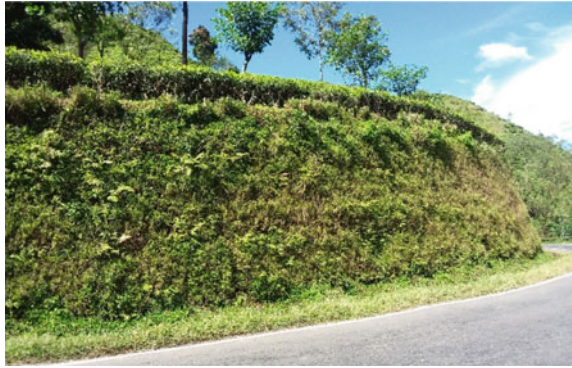
Fig. 16.12 Standing of almost straight earth cut in completely weathered rock with vegetative growth
