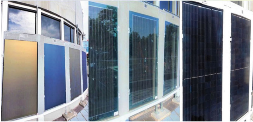
Fig. 3 Photographs of sample BIPV installations on the facade at the School of Design and Environment, National University of Singapore (NUS). (From left) Non-transparent colored BIPV panels, semi-transparent modules, and all-black modules. Reproduced from the BIPV brochure; Copyright 2014, SERIS
