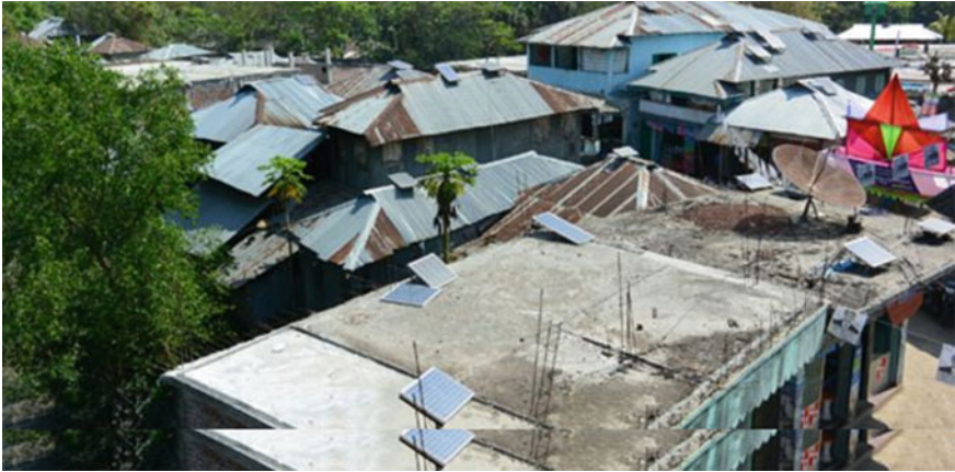
Fig. 8 SOLshare community microgrid in Bangladesh
