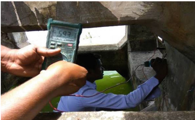
Fig. 6 Half-cell potential test in progress in a RC column of the berthing dolphin of the STB jetties
