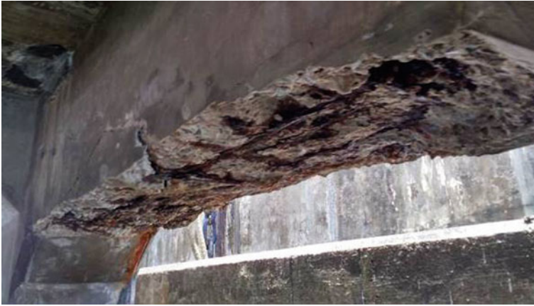
Fig. 4 View of the spalling of concrete noticed in the RC top deck beam of the berthing dolphin 1
