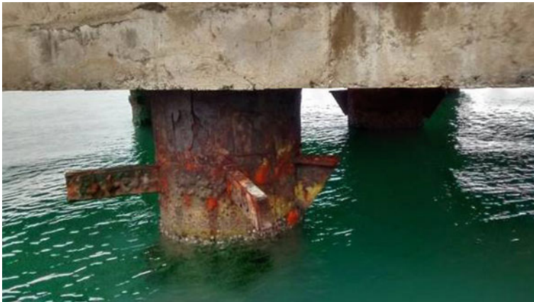
Fig. 9 View of the damaged steel liner of the piles of dolphin 1 of the coal jetties 1
