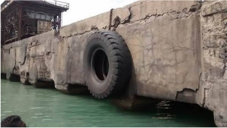
Fig. 10 View of distressed front portion in the jetties head of coal jetties 1
