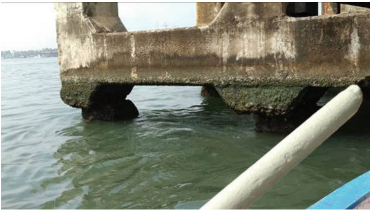
Fig. 5 Mis-alignment was noticed at the junction of the pile haunch and the bottom beams in some of the locations causing a significant eccentricity in the berthing dolphin 1
