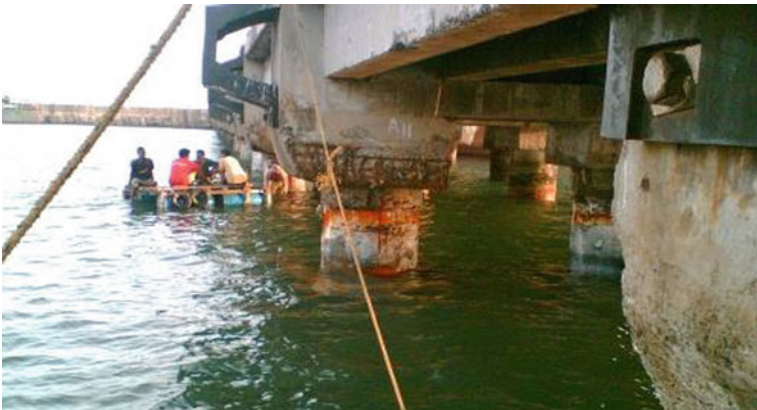
Fig. 12 View of the corrosion affected finger jetties before rehabilitation
