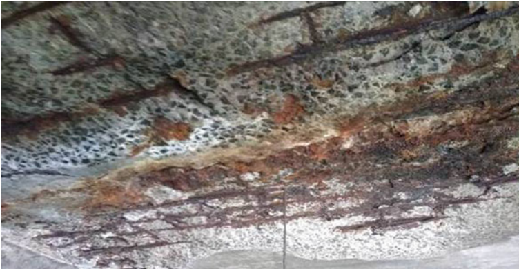
Fig. 2 View of the spalling of concrete with exposure and loss in diameter of rebars in the RC deck slab in the central platform
