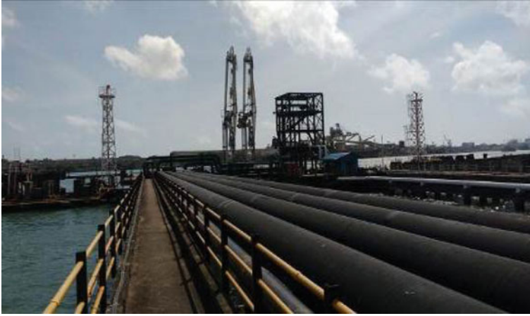
Fig. 1 General view of the NTB jetties at M/s Cochin Port Trust, Kochi
