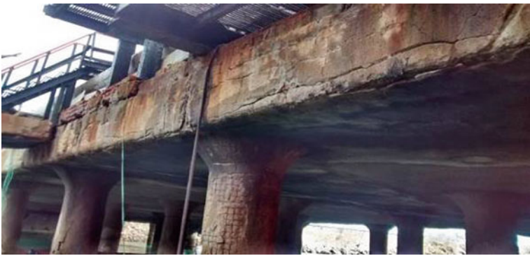
Fig. 11 View of distressed sides in the jetties head of the oil jetties
