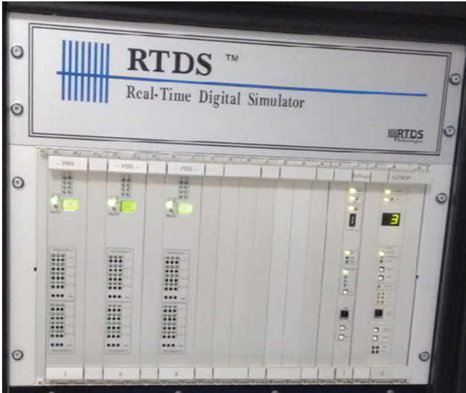
Fig. 3 Close-up front view of one rack
