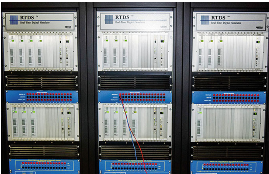
Fig. 2 RTDS front view at IIT Kanpur
