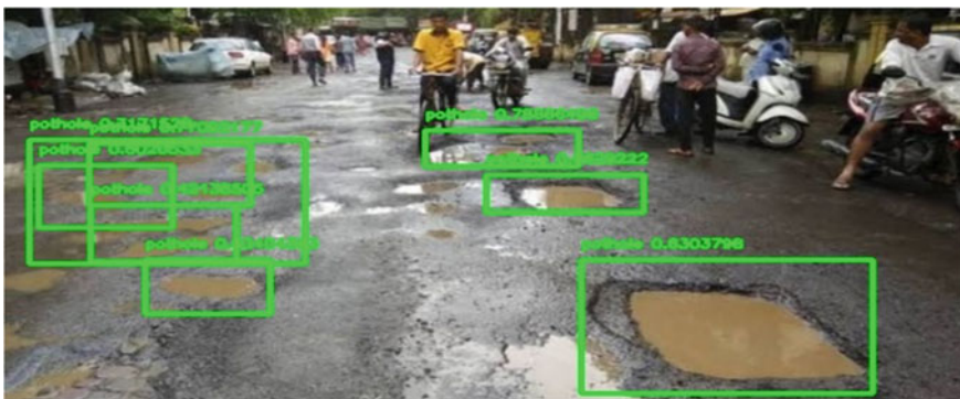
Fig. 3 Multiple potholes detected in an image
