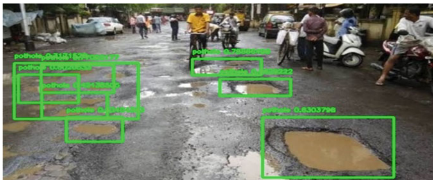
Fig. 3 Multiple potholes detected in an image
