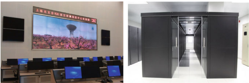
Fig. 5 VLBI data center and server room. Left: Centrally control hall, Right: Server and network device room
