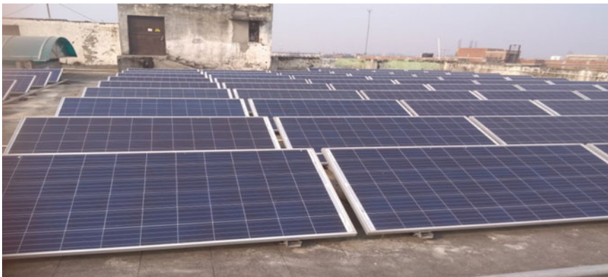
Fig. 1 Installed grid-connected rooftop system
