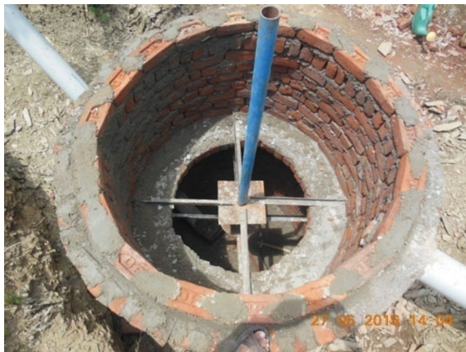
Fig. 3 Top view of modified biogas plant
