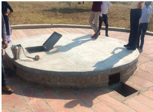
Fig. 20.5 A protected water harvesting structure in Rajasthan (India)
