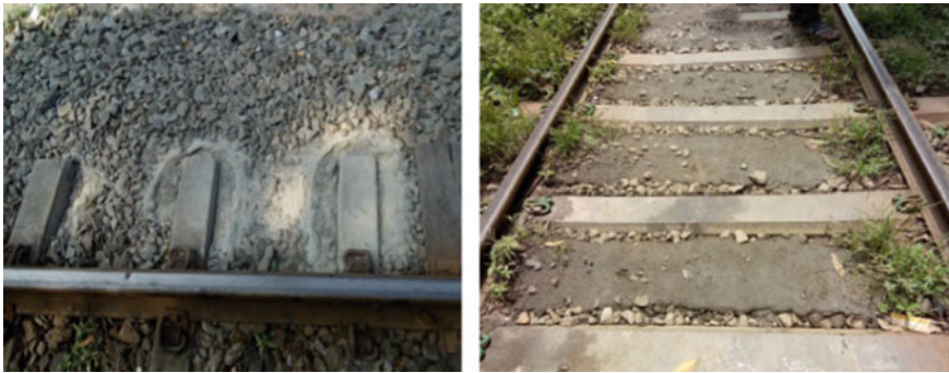
Fig. 1 Degraded ballast railway track
