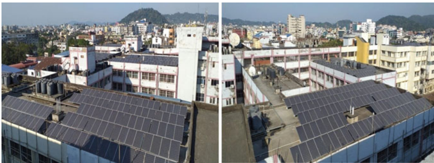
Fig. 2 Picture of 500 kWp grid-tied rooftop PV unit
