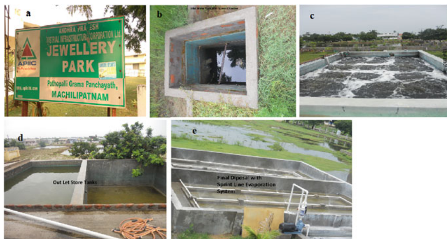
Fig. 1 a Jewellery Park Entrance, Pothepally, Machilipatnam. b Inlet water tank with screen chamber. c Equilization tank. d Outlet store tank. e Final disposal outlet tank
