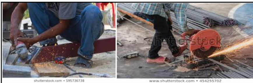
Fig. 2 Unsafe work behavior of worker
