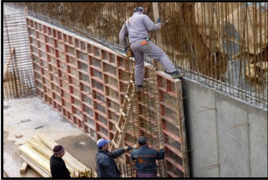
Fig. 3 Unsafe work behavior of workers
