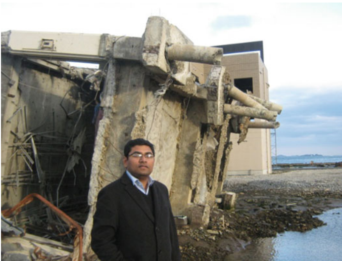
Fig. 10 Collapse of the pile-supported building following the same earthquake
