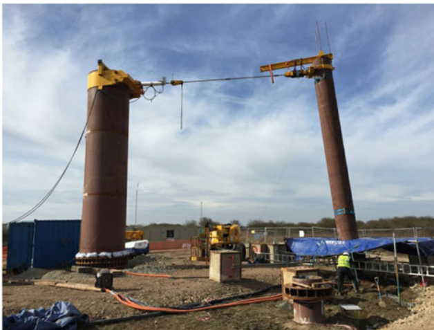
Fig. 18 Set up for testing of lateral capacity of monopiles (Byrne et al. 2015)
