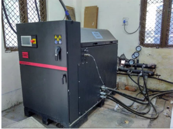
Fig. 7 Hydraulic power unit (HPU)
