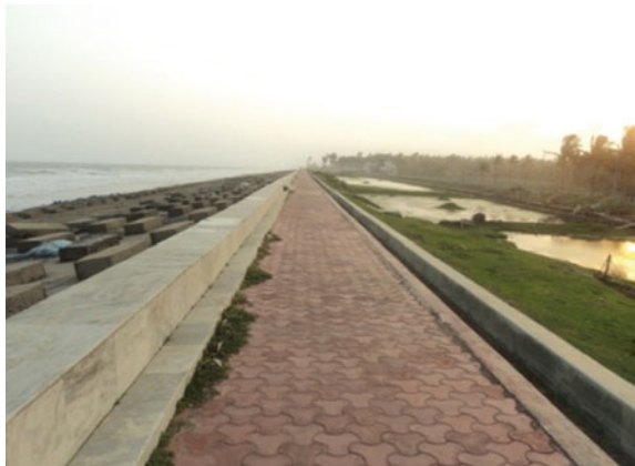
Plate 6 Water over flow at land
