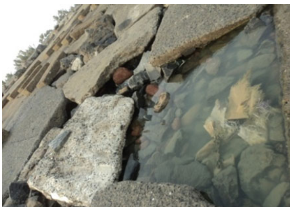
Plate 4 Wave overtopping of seawall
