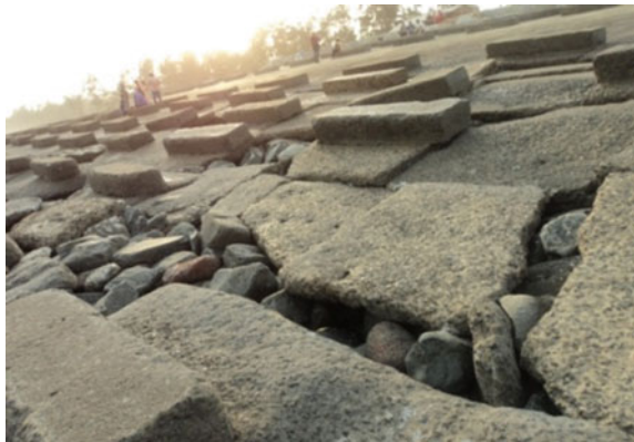
Plate 1 Collapsing seawall at Shankarpur
