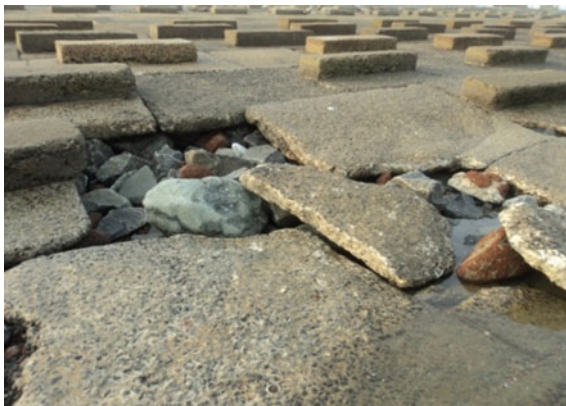
Plate 2 No repair work of seawall
