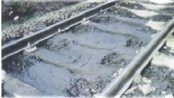
Fig. 3 Mud pumping (sourced from Lieberenz et al. 2009)
