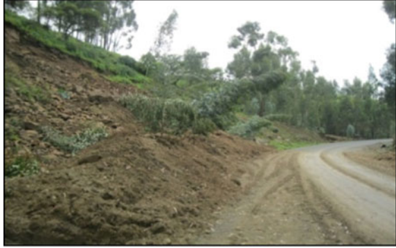
Fig. 4 Landslide from hill slope along “Kombolcha–Mekane Selam”
