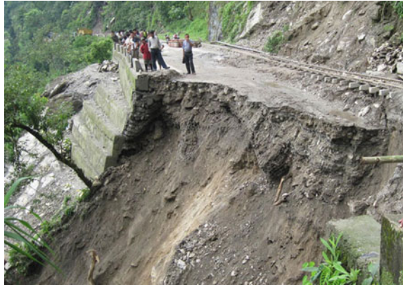
Fig. 2 Landslide damages in Paglajhora region ( Source Save The Hills )
