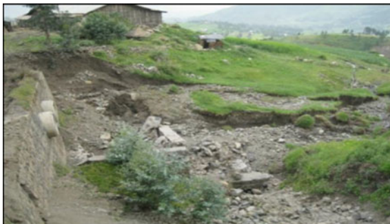
Fig. 6 Landslip of d/s side valley slope at pipe culvert location along “Kombolcha–Mekane Selam”
