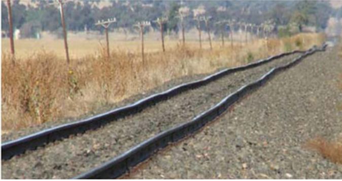
Fig. 2 Differential settlement of track (sourced from Suiker 2002 )
