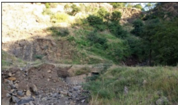
Fig. 7 Landslip at slab culvert location along “Adiremet–Dejena–Dansha”
