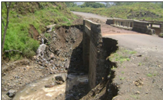
Fig. 2 Landslip from bridge approach slope along “Adiremet–Dejena–Dansha”
