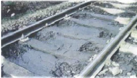
Fig. 3 Mud pumping (sourced from Lieberenz et al. 2009 )
