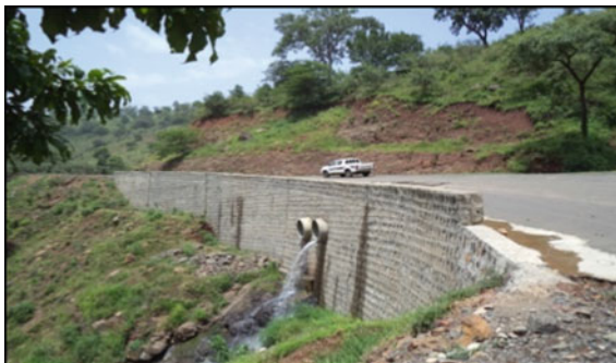
Fig. 17 SM head wall cum retaining wall done at pipe culvert locations in Ethiopia
