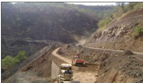
Fig. 19 Typical photograph of restoration measures of valley slope along project roads in Ethiopia
