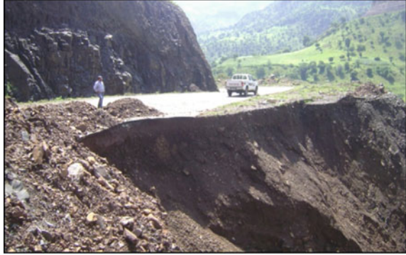
Fig. 8 Landslide of valley side slope along “Adiremet–Dejena–Dansha”
