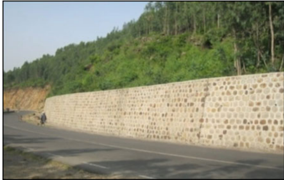
Fig. 16 Provision of stone masonry retaining wall at toe of hill slope in Ethiopia
