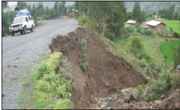
Fig. 9 Landslide of valley side slope along “Kombolcha–Mekane Selam”
