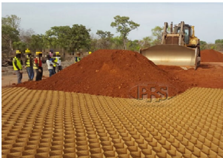
Fig. 15.10 Installation and infill of Neoloy Geocell on rural feeder road project. Photo Credit UNOPS
