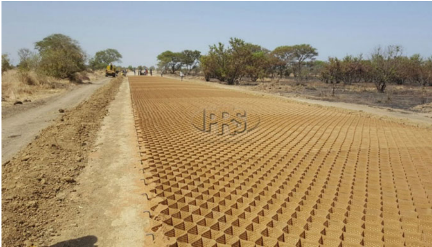
Fig. 15.7 Installation of Neoloy Geocell on rural feeder road project, UN. Photo Credit UNOPS
