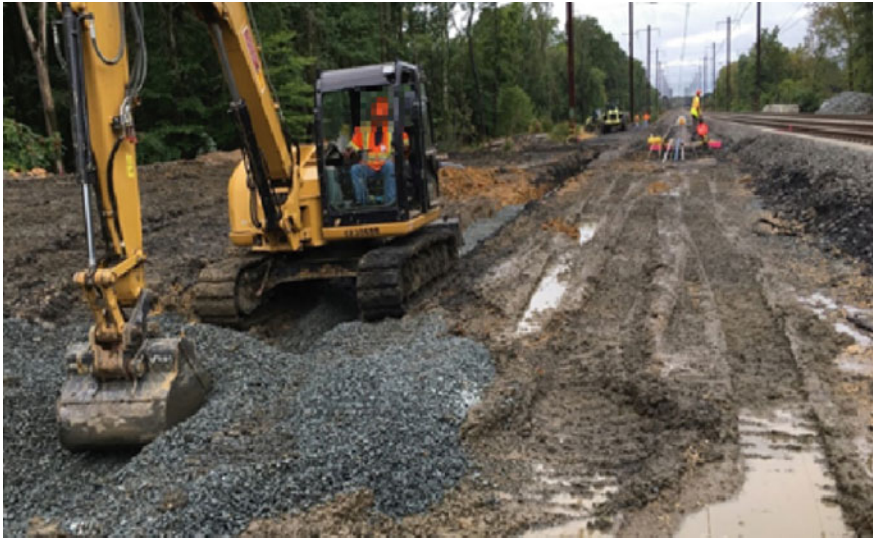
Fig. 15.12 Poor clay subgrade conditions on Track C (before rebuild). Photo Credit PRS Geo-Technologies
