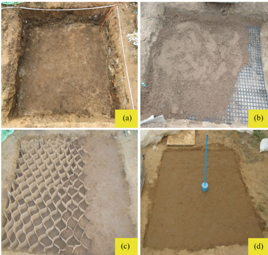
Fig. 8.7 Preparation of foundation bed: a Excavated test pit; b Partially filled geogrid; c Partially filled geocell pockets; d Levelled foundation bed. Source from Venkateswarlu et al. (2018)
