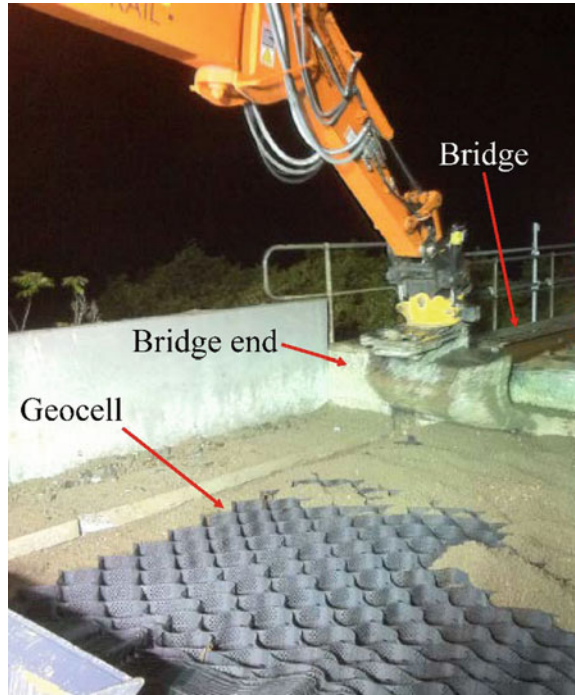
Fig. 11.8 Installation of geocells at the railway bridge ends on the south coast line of New South Wales, Australia. Modified from Kaewunruen et al. (2016)
