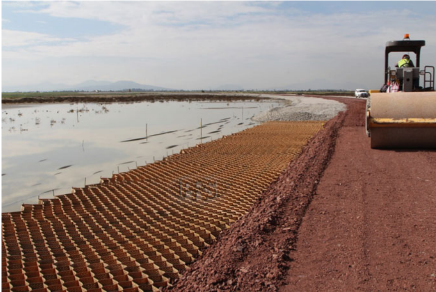
Fig. 15.5 Compaction of volcanic rock infill, during installation of NPA Geocell in swampy soil. Photo credit Innovater
