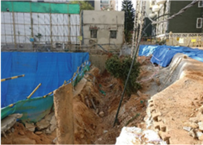
Fig. 2 Photograph of the failed section
