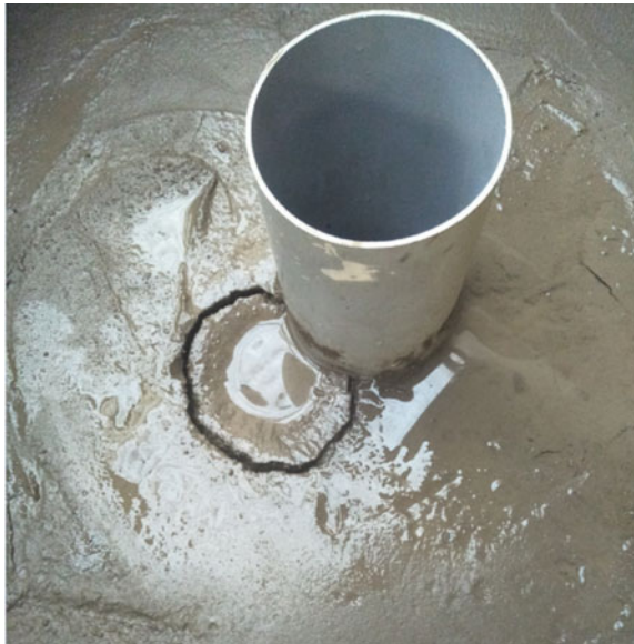
Fig. 2 Subsidence in model
