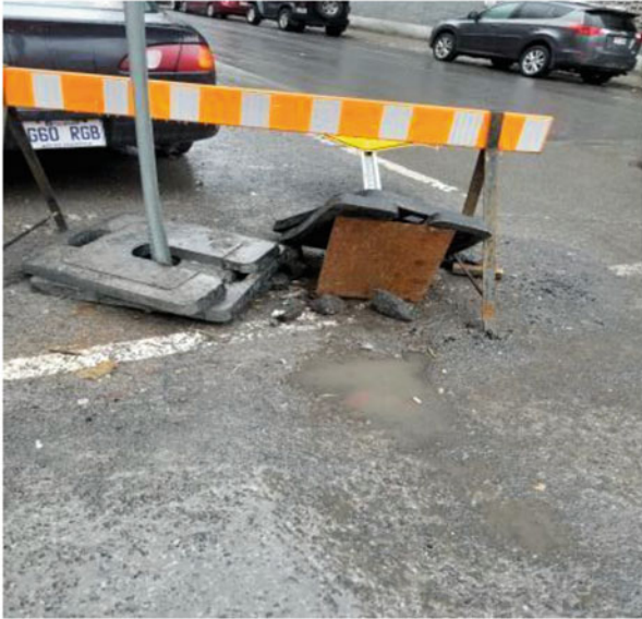
Fig. 7 Open, unattended construction site on pedestrian pathways
