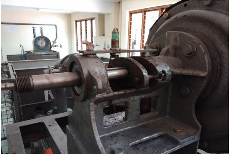
Fig. 3 Turbine—dismantled for measurements
