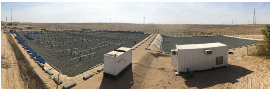
Fig. 7.2 An aerial overview of the two-stage constructed wetland facility just before the completion of the construction phase. (Courtesy of Bauer Nimr LLC)
