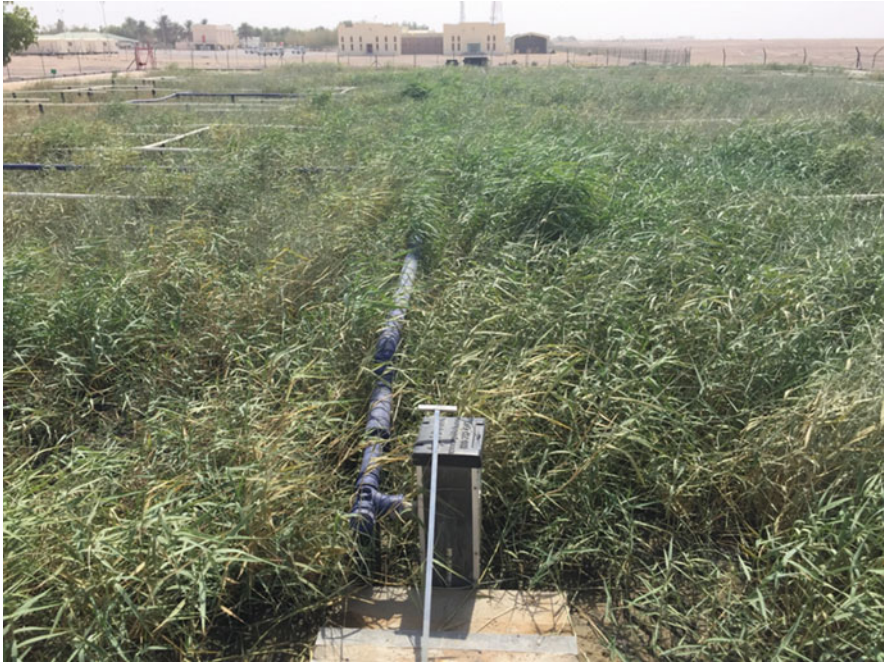
Fig. 7.3 The first-stage vertical flow constructed wetland for sludge mineralization during operation. (Courtesy of Bauer Nimr LLC)
