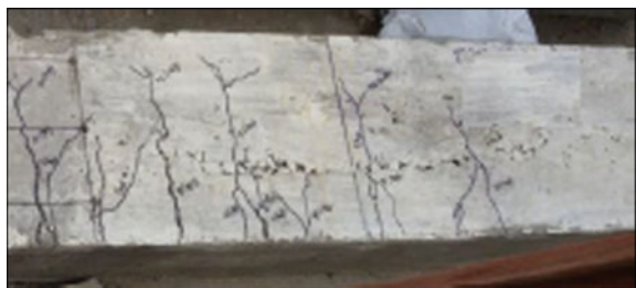
Fig. 7 Cracking pattern for control beam CBF
