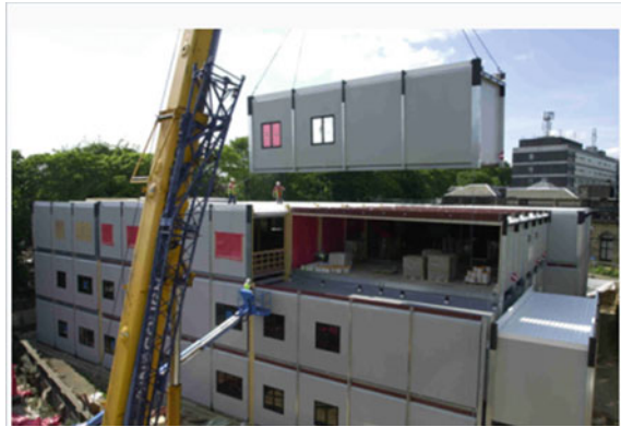
Fig. 10 Non-load-bearing modules placed into a primary frame structure. (Source Steel Construction. info)
