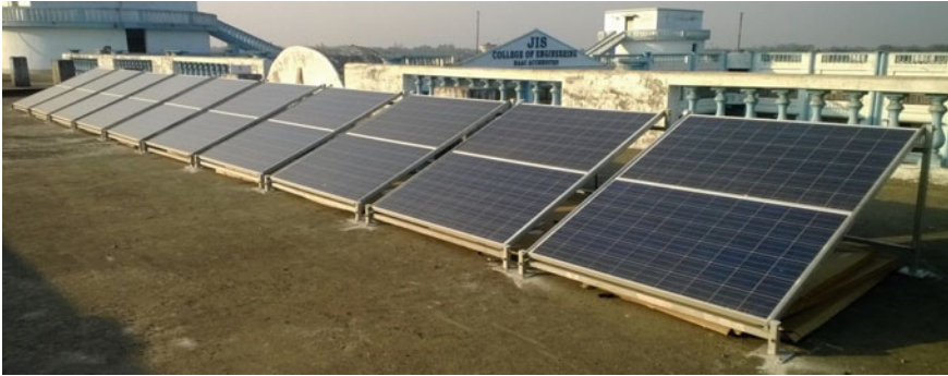
Fig. 1 Solar photovoltaic power plant at JIS College of Engineering
