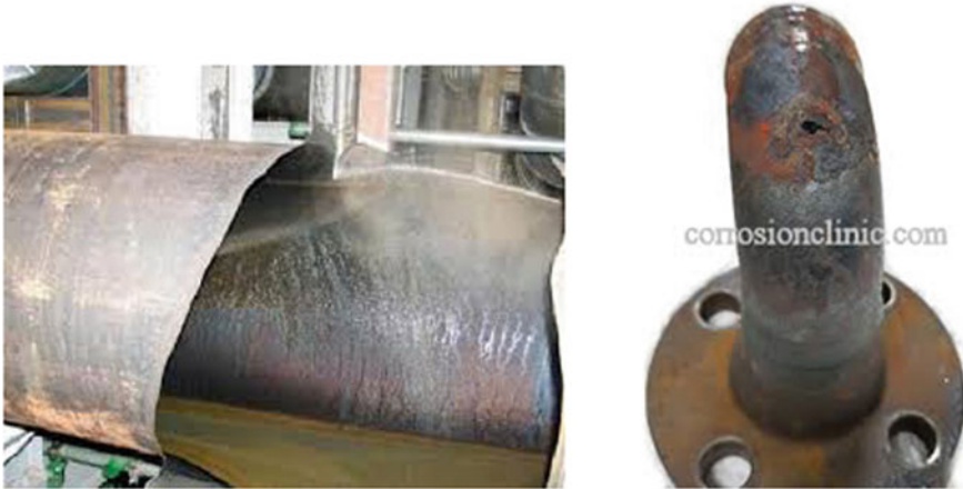
Fig. 12 Failure of piping material due to flow assisted corrosion
