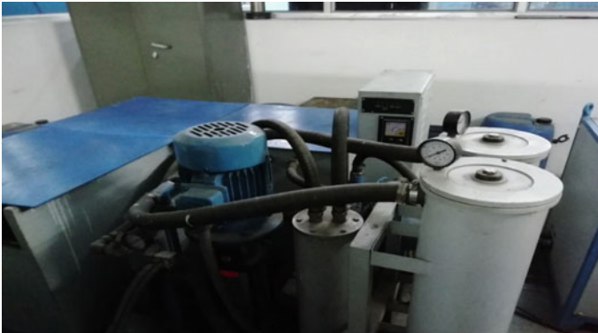
Fig. 27.3 Dielectric flushing unit
