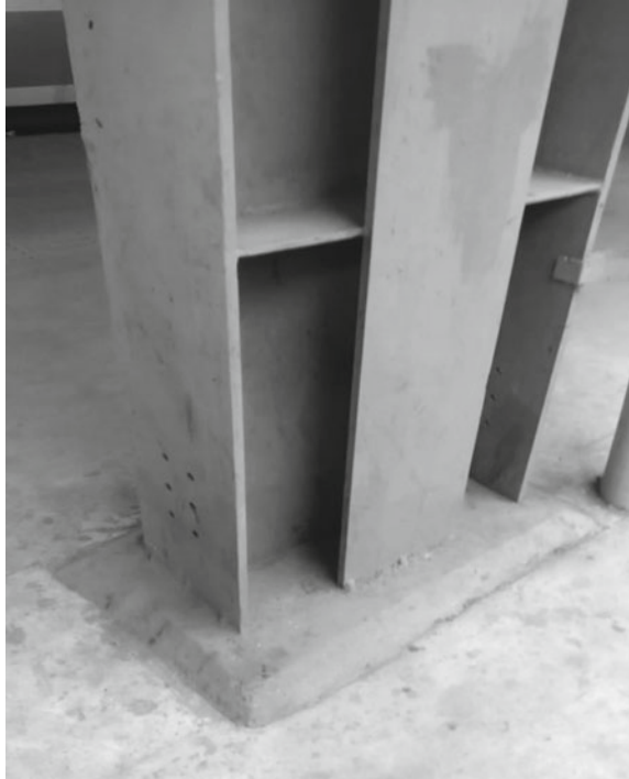
Fig. 1 Image of lower portion of column observed at Andheri station
