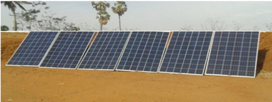
Fig. 2 Solar photo-voltaic array (six panels)
