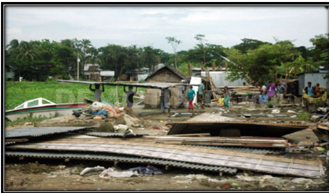
Fig. A.1 Shifting of housing structure
