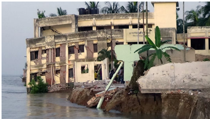
Fig. A.2 Padma River erosion at UpaZila Health Complex Naria, Shariatpur. Source: www.thedailystar.net
