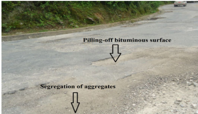
Fig. 3 Pilling-off bituminous layers and segregation of coarse aggregates and bitumen on Thimphu–Trashigang Highway. Courtesy of Mr. Karma Dorji, Deputy Executive Engineer, Lobesa
