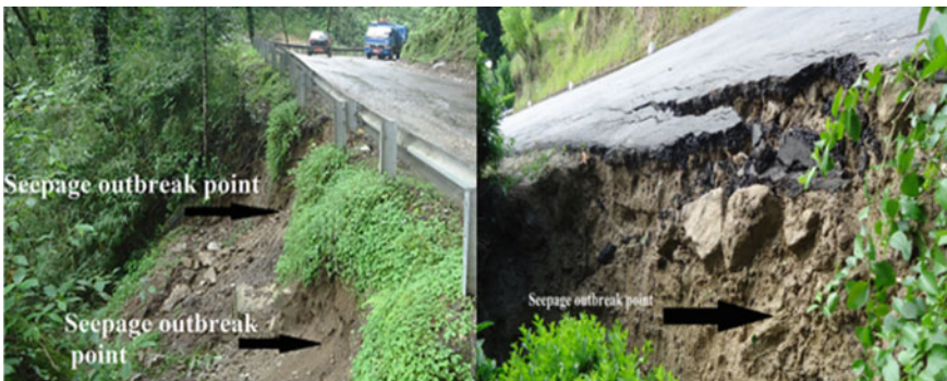
Fig. 2 Sliding of road edges due to uncontrolled seepage in subgrade soils or surface run-off from road surface on Thimphu–Trashigang Highway. Courtesy of Mr. Karma Dorji, Deputy Executive Engineer, Lobesa
