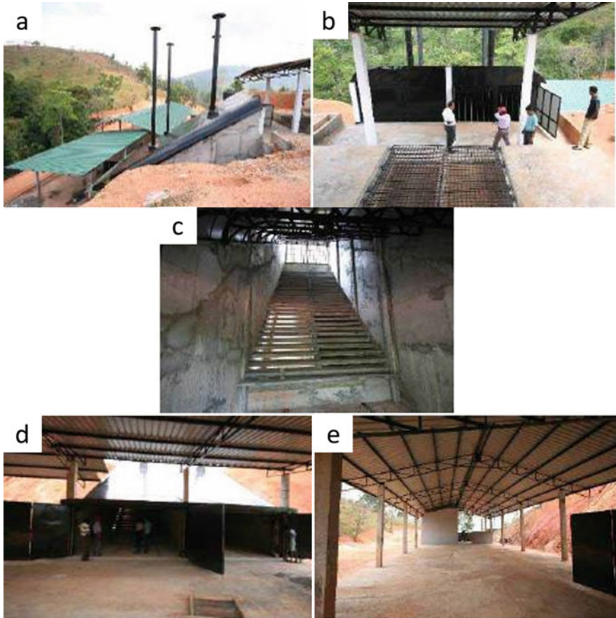
Fig. 6 ISG unit at Nawalapitiya UC. (a) Overview, (b) inlet of ISG for waste, (c) Inclined Step Grates, (d) outlet of ISG and (e) maturation yard
