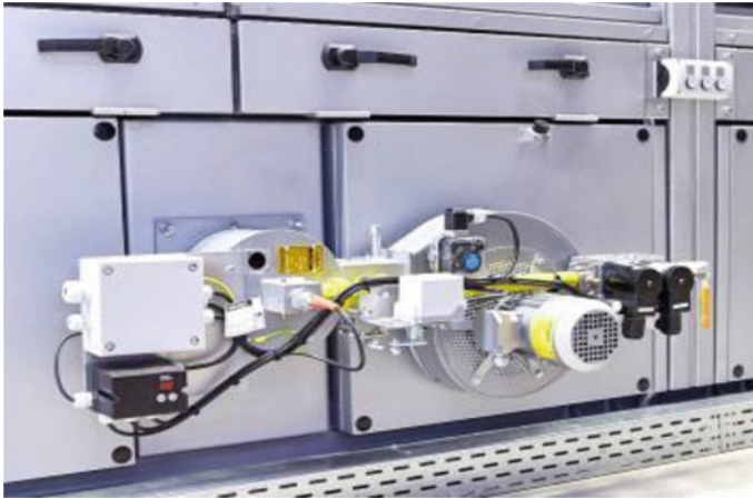
Fig. 51 Gas fired system
