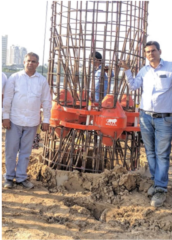
Fig. 2 Installation of S-Cell assembly in cage of diameter 1.5 m for test pile at foot over bridge construction in Sabarmati Riverfront Ahmedabad, Gujarat, India
