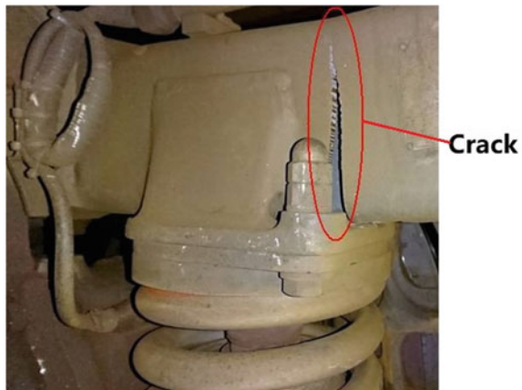
Fig. 1 Crack in bogie system of the Shinkansen
