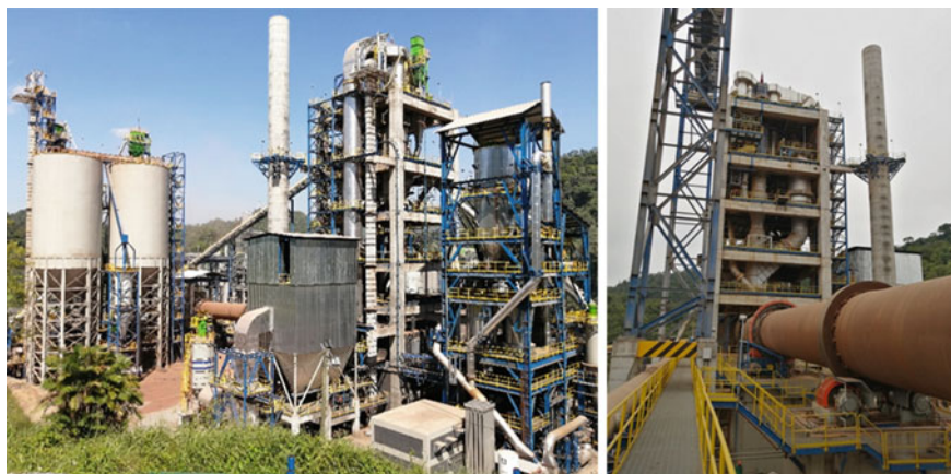
Fig. 4 Industrial plant with flash dryer–rotary kiln system
