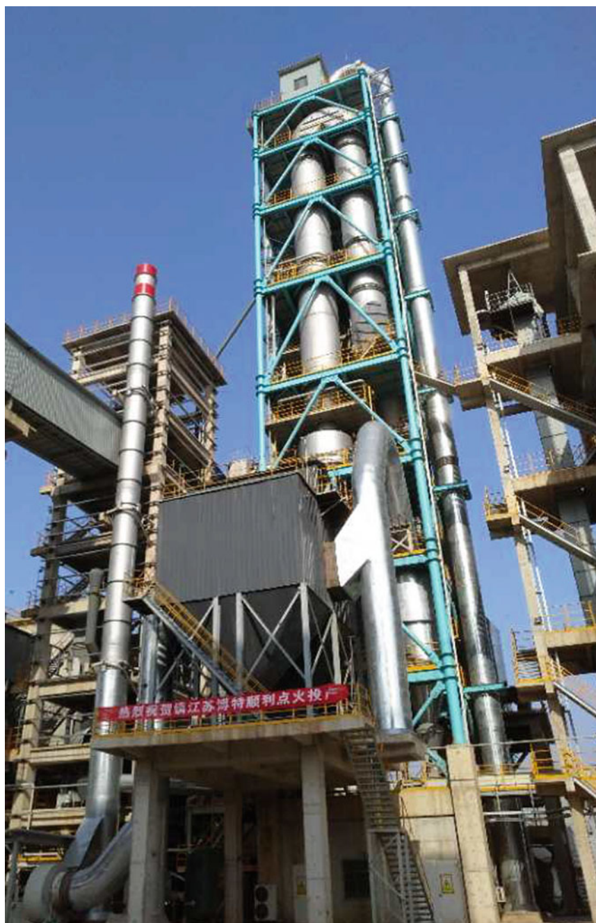
Fig. 3 Demonstration production line of suspension calcining and cooling system
