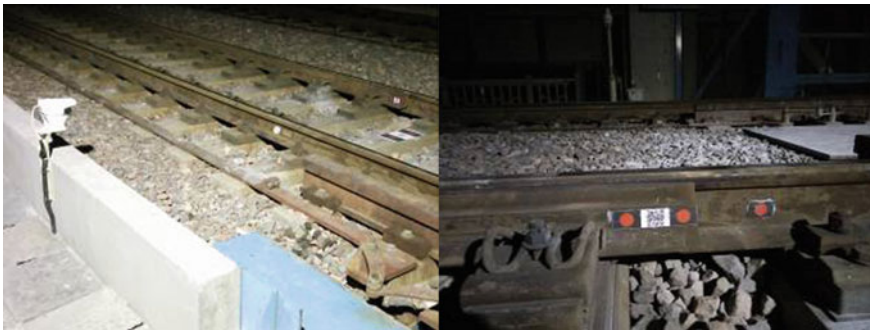
Fig. 7 Actual point of switch rail displacement monitoring
