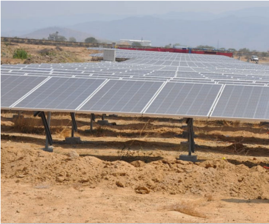
Fig. 4 Ground-mounted solar PV plant at Renigunta Airport, Tirupati
