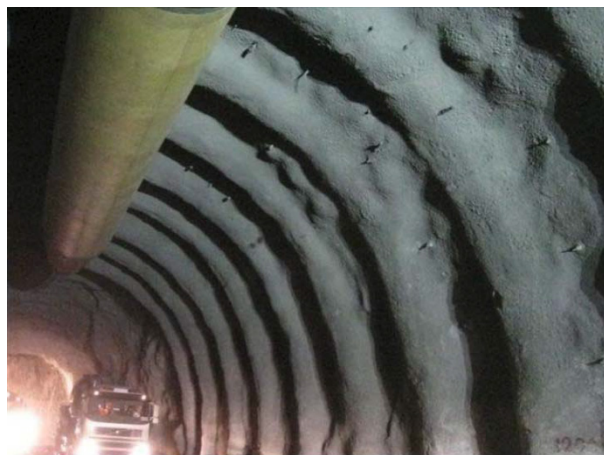
Figure 5. Finished product showing tunnel support with RRS in a tunnel in Oslo (NPRA, 2010)
