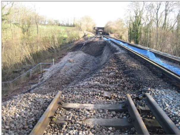
Figure 15. Stonegate slip on the London to Exeter line, UK, in February 2014 (photo: @networkrail)
