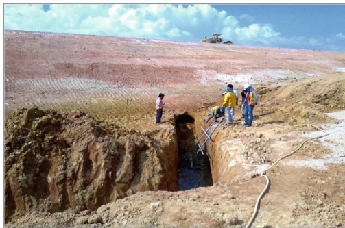
Fig. 4. Concentrated leak at left abutment of existing dam.
