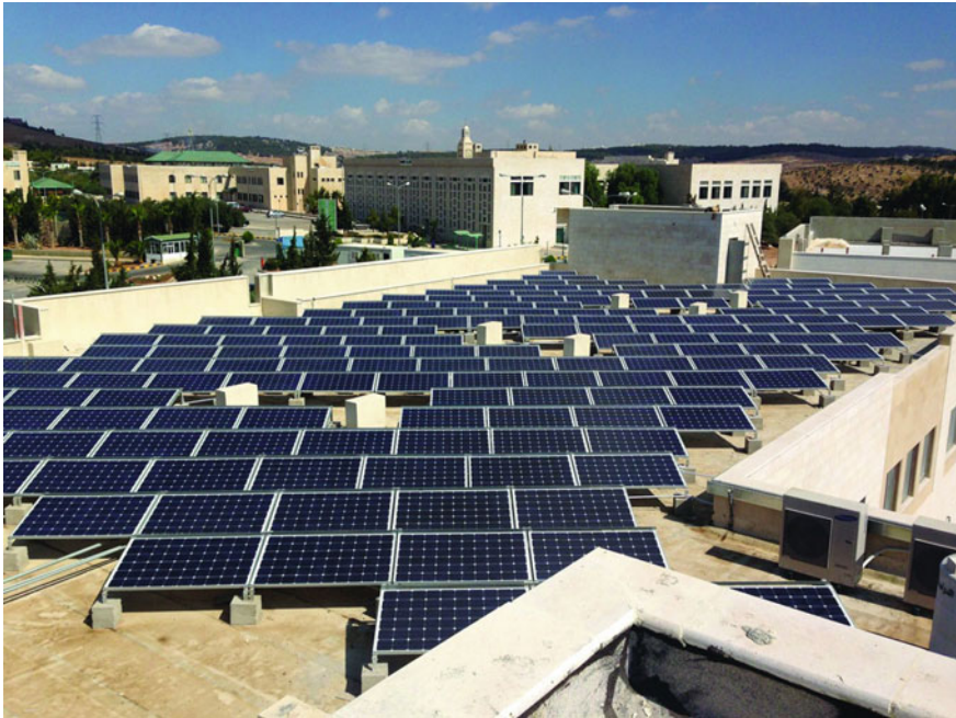
Fig. 1 Solar panels mounted on building roofs
