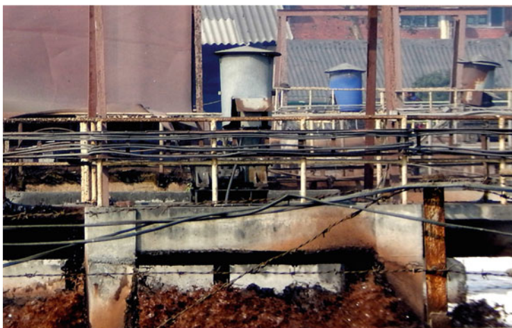
Fig. 1.5 A view of the aerated activated sludge treatment of pulp and paper industry wastewater
